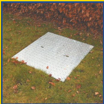
CLF1 - 6pe Fully Installed.
