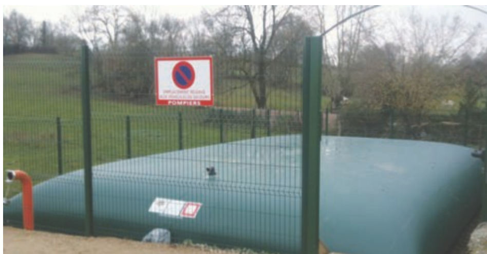
120m 3 fire protection tank with INC14 in a housing estate
