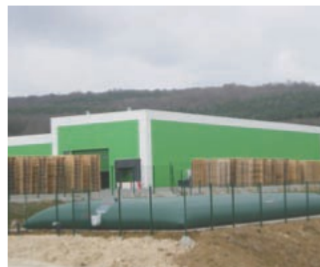
240m 3 fire protection tank with INC14 in an industrial zone
